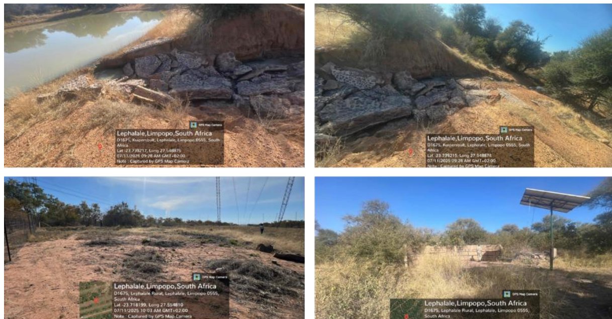
Figure 17: Top left and Right -Collapsed bridge infrastructure of the existing Impala dam; Bottom left – Servitude on site; Bottom right – Borehole with a solar panel.
